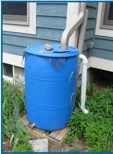
A rain barrel installed at a Brighton home.
